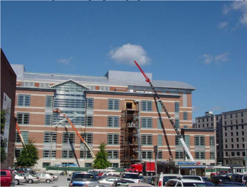
Figure 1. The Worcester Trial Court under construction with finished metal roofing in place
